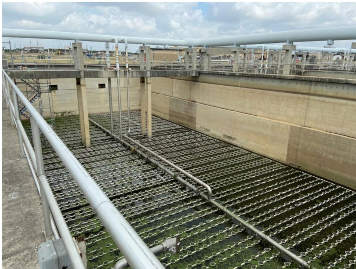
Aeration Basin (Empty)
