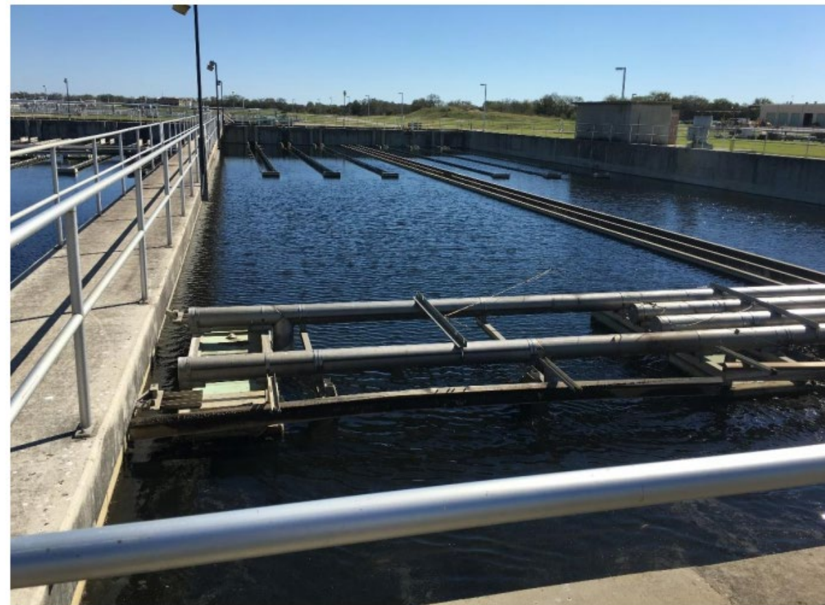
Rectangular Settling Tank
